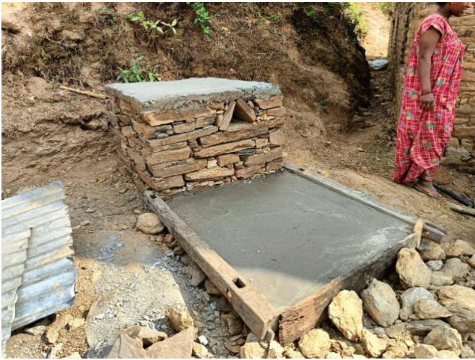
Water point being constructed for the earthquake-affected family in Bheri Municipality, Jajarkot.
