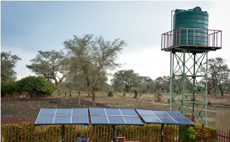
The mechanised water system is made up solar panels, pipes, pump, tank and switch.
